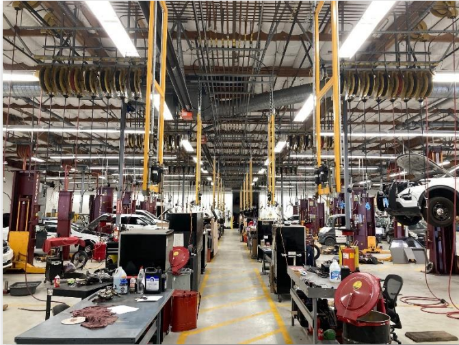
Employee Safety - 10' Clearance Between EV and Closest Metal Object Possible?
