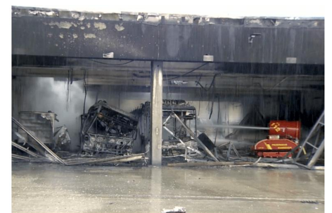
EV Bus Fire Damages Depot Germany, 2021
