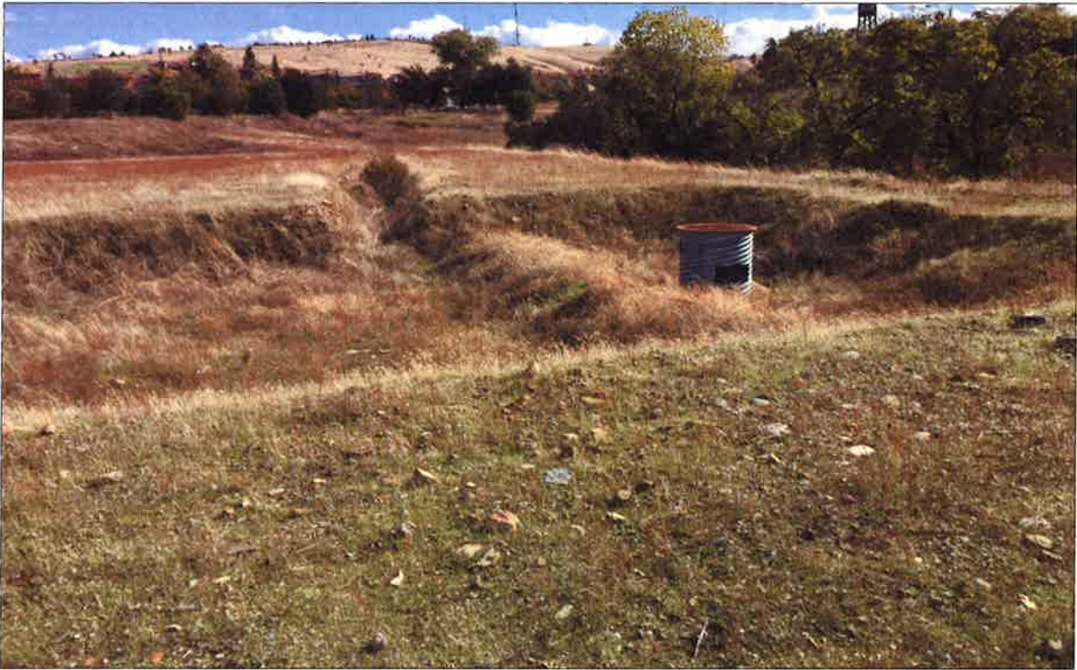
Photo 3. Looking northeast at the drain for the perimeter ditches in the southwest corner of project site
